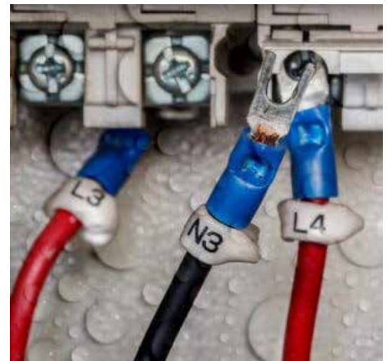
Summer humidity can cause short circuits when cooling equipment if set up wrong
